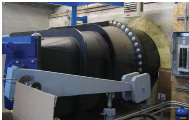
7. New Horizontal Turbine (blue section) recently installed at Royal Mill, West Warwick
