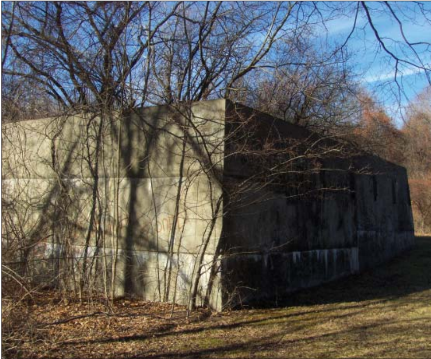
13. Elevated Settling Tank
