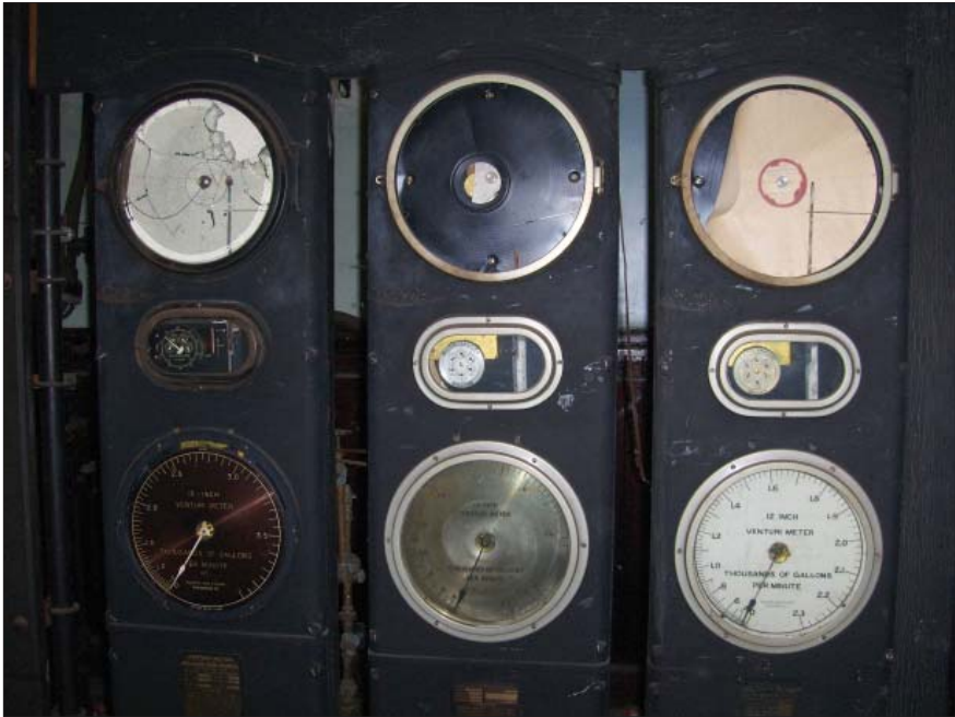
8. Pump House: Meters for Measuring Flow Rate
