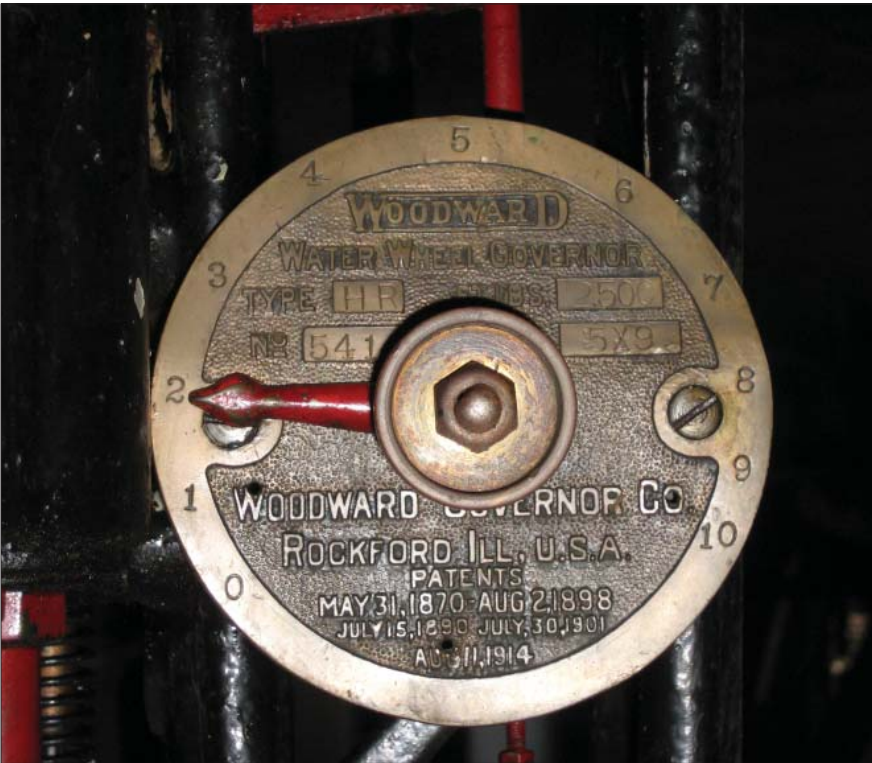
10. Pump House: Water Wheel Governor
