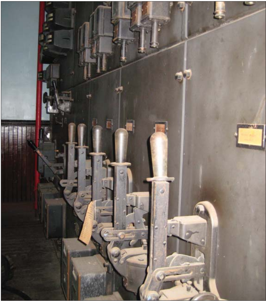
7. Pump House: Electrical Switching Gear
