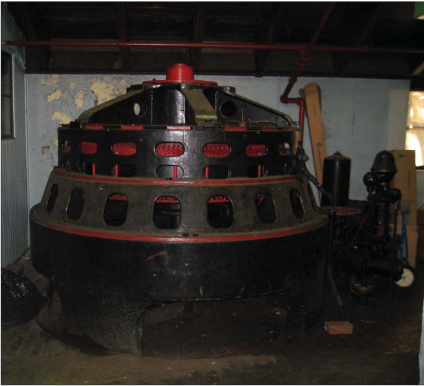
9. Pump House: Alternator (c. 1930)
