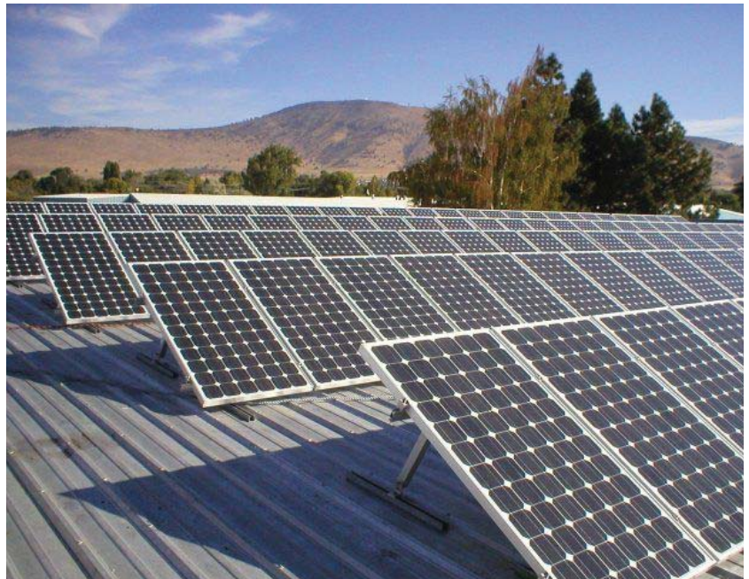
8. Example of Photo-Voltaic Array
