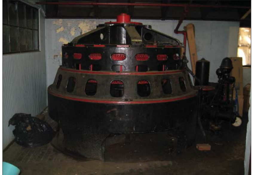
5. Existing Alternator in Pump House (circa 1930)
